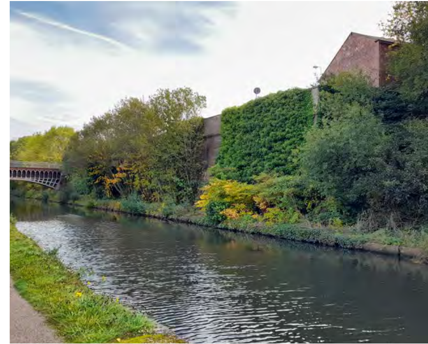
Retaining wall to the Corporation Yard along the New Main Line (Grade II listed)
